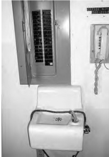
Photo of an old electrical panel with a wall-hung drinking fountain directly below it and a wall phone to the right of it.
